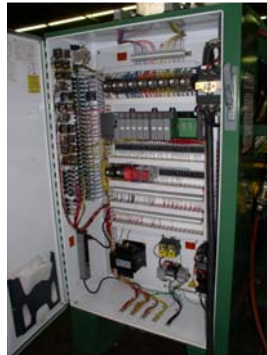
Allen Bradley electrical controls include the SLC 503 series Processor.
